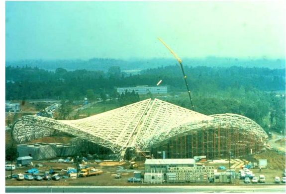
Roof of concert hall consisting of two fan-shaped hyperbolic paraboloidal double layer steel structures, length of each fan about 80 m, capacity: 3000 people, Tsukuba, Japan, 1985, Tomoe Corp
