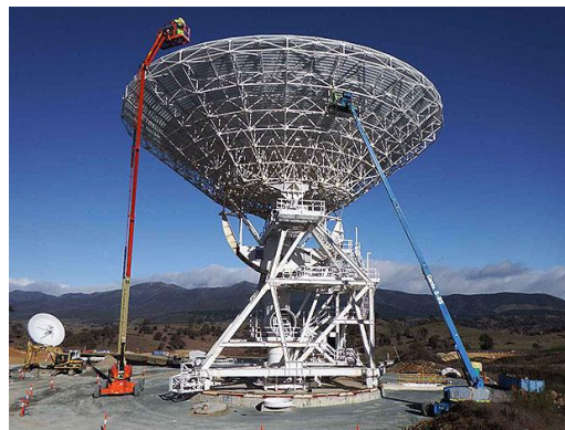
Deep Space Station 35 (DSS35) is a new antenna being built at the Canberra Deep Space Communication Complex (CDSCC) at Tidbinbilla, southwest of Canberra, Australia
